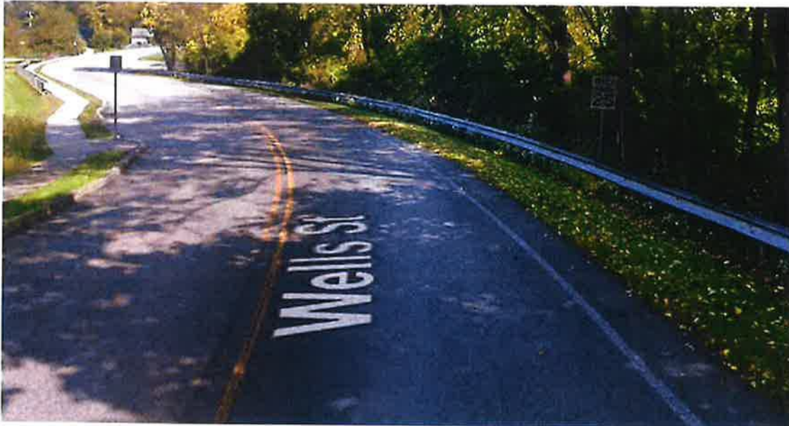
Figure 2 Speed Limit Sign on Wells needs to be replaced
