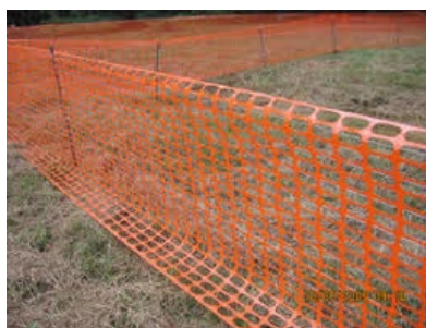
Fencing protects areas from compaction
