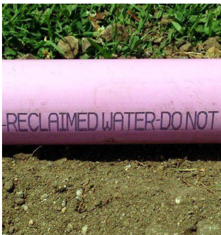
Purple pipe for recycled water.
