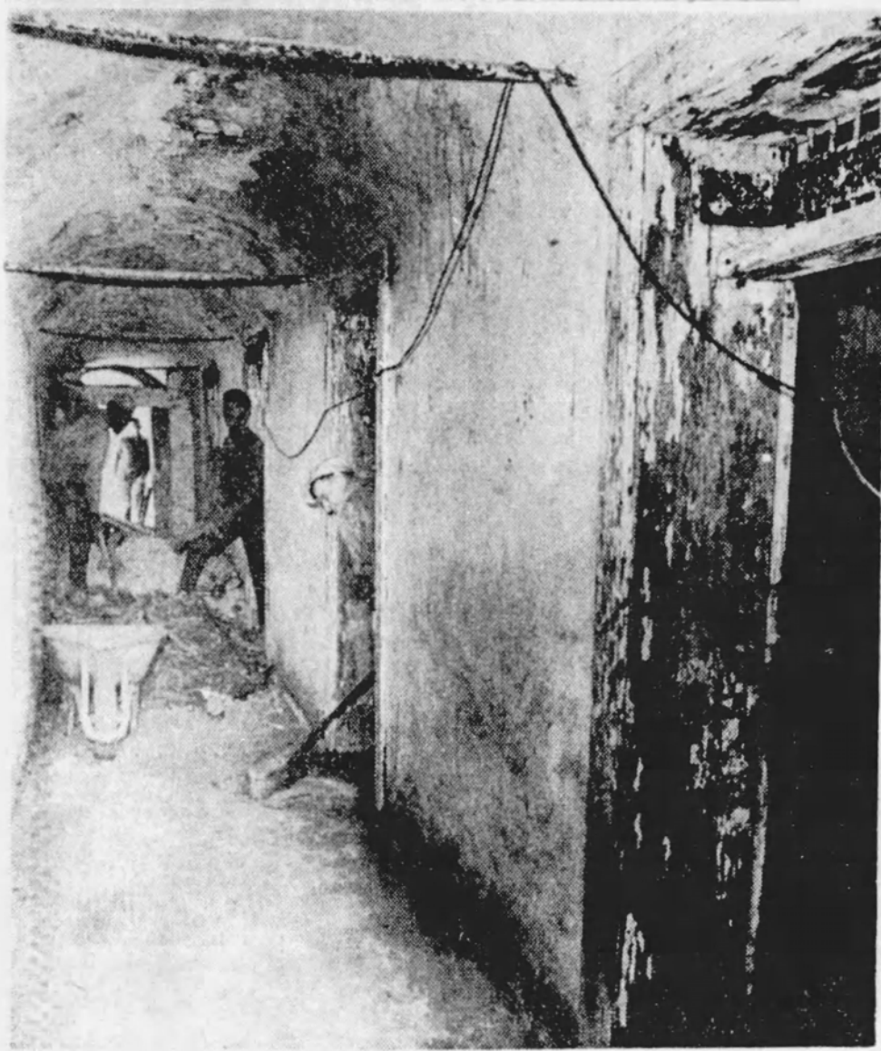
Workmen are shown tearing up the rotted wooden floor and clearing debris in the process of restoring the old dungeon below the old Market House in Columbia. At left is shown the long, narrow tunnel with its vaulted ceiling. The doors on the right lead to cells. Over the door is an iron grating which was the
