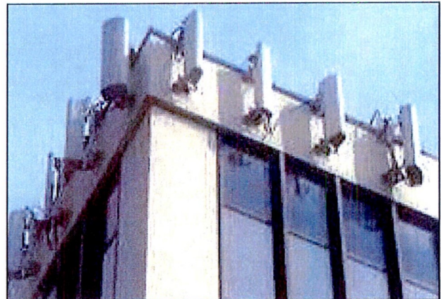
The antennas are not concealed and interrupt the architectural theme
