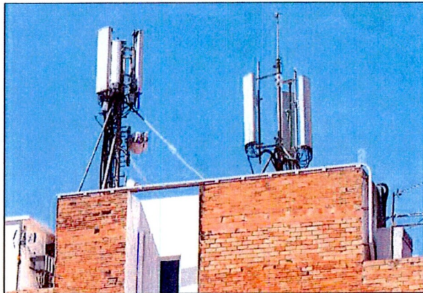
The antennas are vertically revealed with no screening
