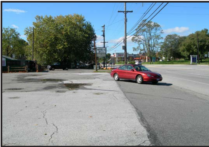
Excessively Wide Curb Cut
