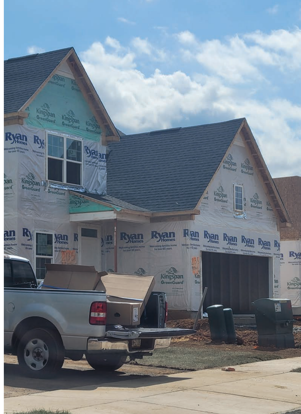
Residential construction at The Estates at Willow Brook. Woodmont Lane, North Catasauqua Borough.
