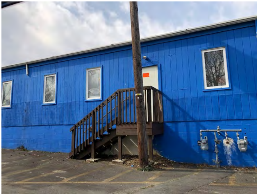
1960 N Olden Ave from Olden Avenue. View along the east side. Stop work orders issued. No use currently permitted in this section of building. Photo taken February 2020
