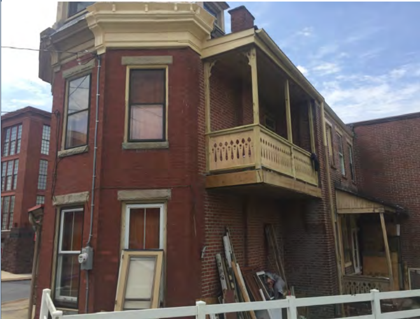
Here is an example of an historic porch rehabilitation project in the Allison Hill historic district. Notice the rails, balustrades, and posts match the original materials and design.
