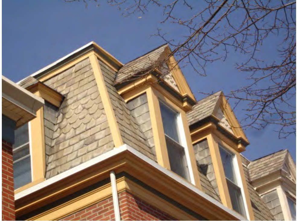
A pair of gabled dormers projecting from a slate Mansard roof. Mansard roofs were usually constructed with built-in box gutters.
