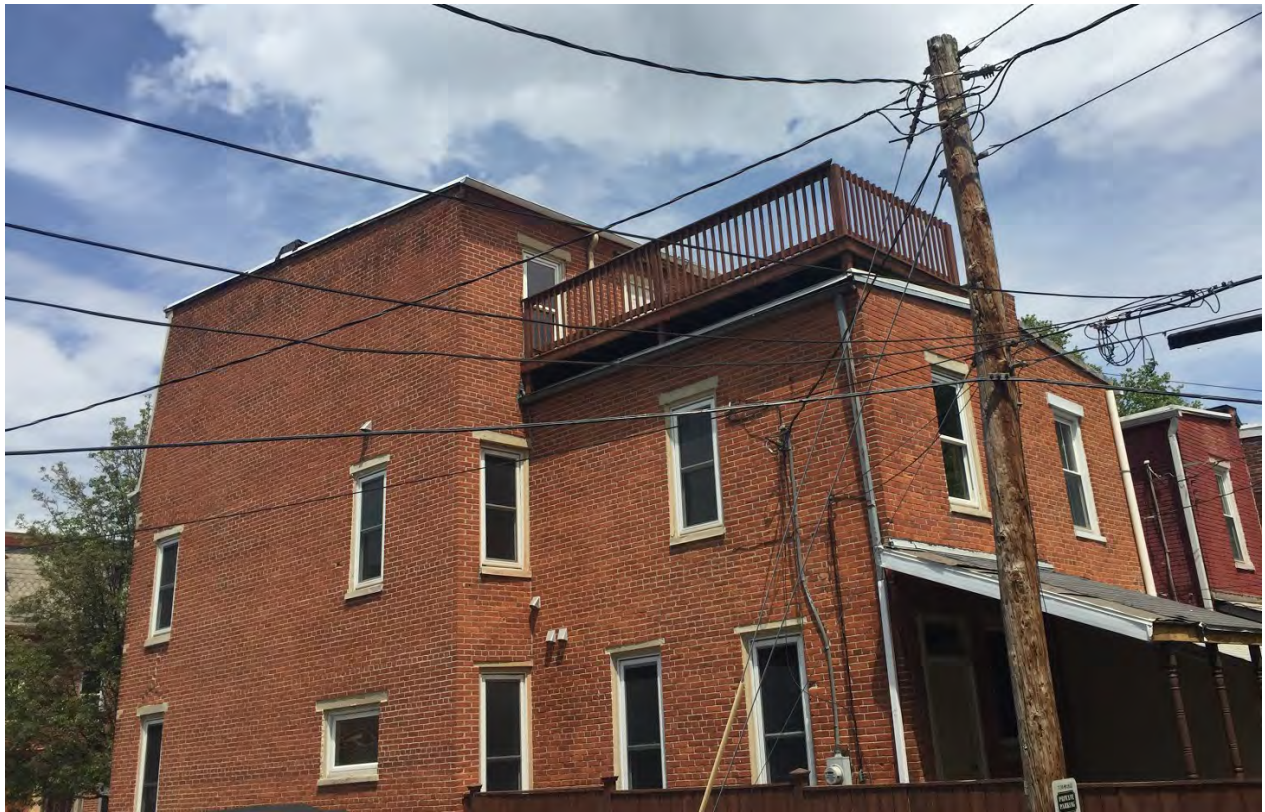
A rooftop deck was recently installed on this Uptown home. Rooftop decks can have an impact on property values. Rooftop decks have a large visual impact on the historic district and usually require HARB review.
