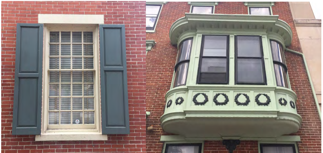
Character defining historic windows should be maintained and repaired as necessary. Replacing curved bow windows or multi-lite windows can be difficult and expensive thus making it important to take preventative measures to preserve them.
