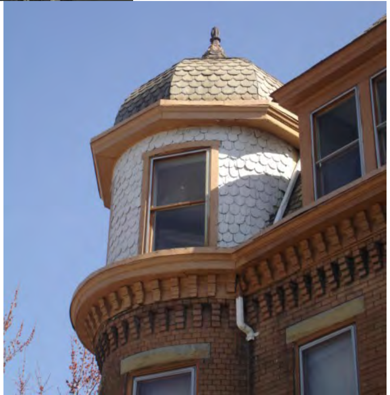
The wooden shingles on this turret have been properly maintained and repaired.
