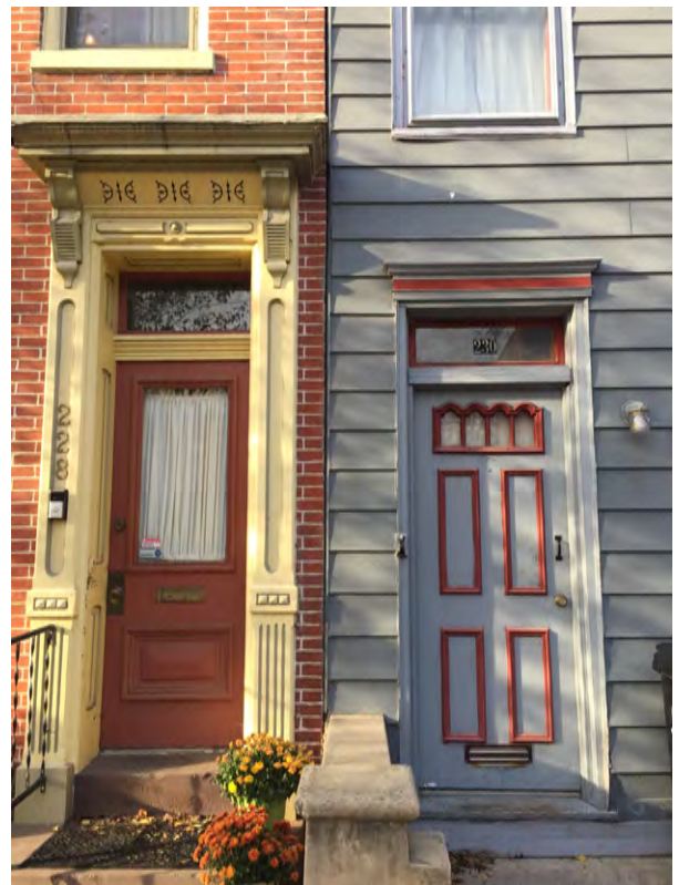
The door and surround on the left has been maintained and preserved whereas the door and surround on the right has been severely altered.
