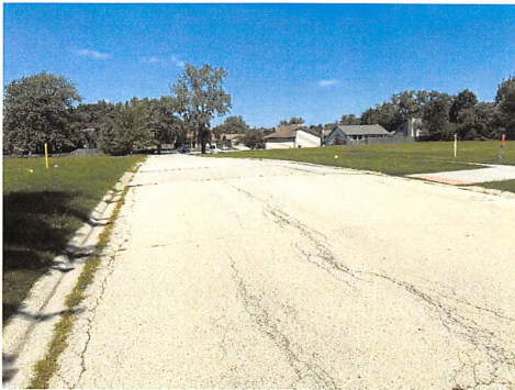
22. Easternmost Project Limits: Proposed trail connection to existing Heroes Trail at Heatherwood Drive, Facing North
