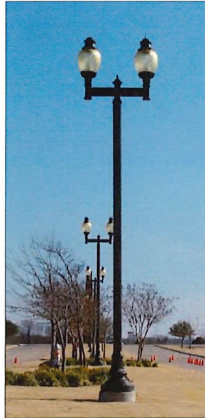
Figure 14: Example Light Pole and Fixture
