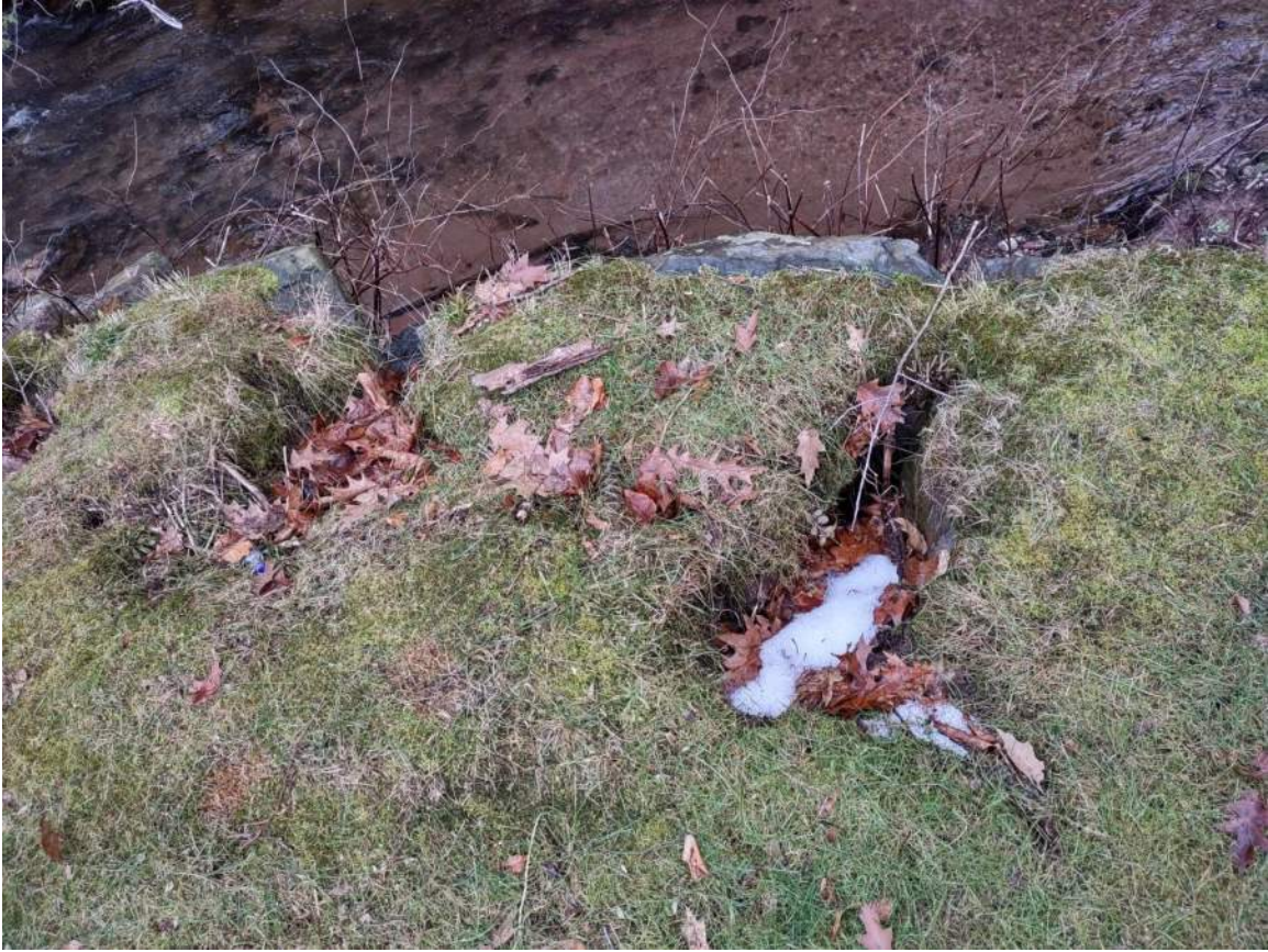
Recent scour (since summer 2021) in between large existing rocks on surface, creates trip hazard
