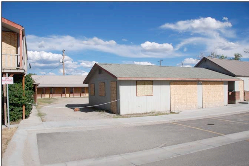
Figure 15: Existing Conditions—the Pine Creek Motel is a classic example of American Roadside Architecture. With the exception of the wood panel clad
