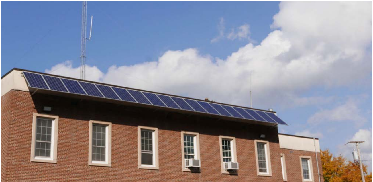
Solar Panels on Village Hall, 2020 by Vanessa Bertozzi
