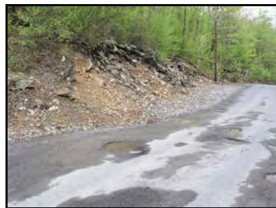
Erosion Problem in Area with Development on Steep Slopes
