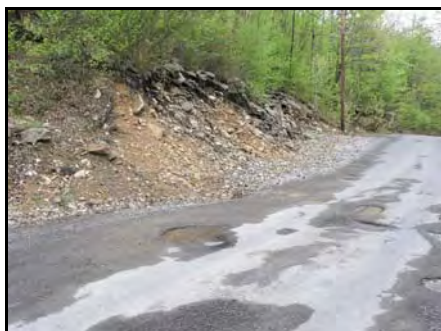
Lack of Stormwater Planning
