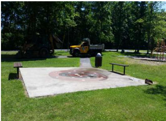
Broken & undersized splash feature
