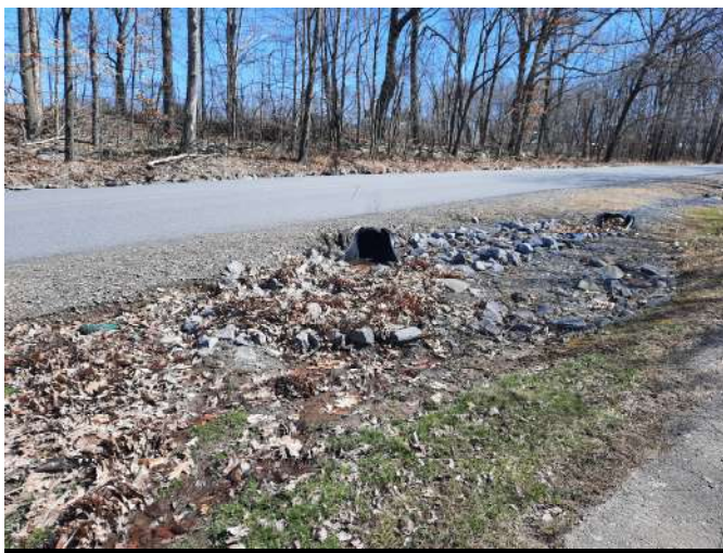
Park Road swale system often overflows
