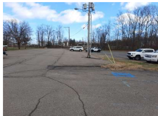
Parking lot is disjointed and inefficient
