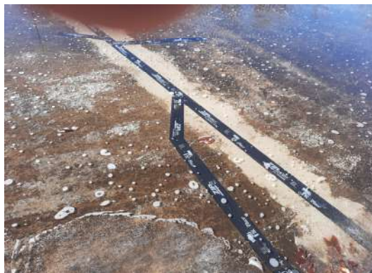
Ice rink cracks recently patched
