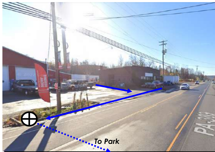
This catch basin along SR-309 directs runoff into the Park Road swale system
